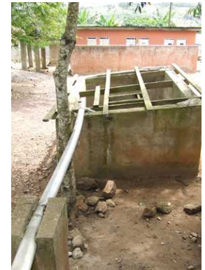
Borehole that provides water for school was built by the RMF
